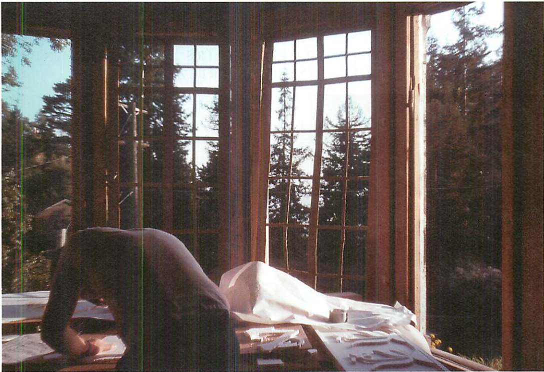
Cardboard mockup to test the size and distribution of glazing bars in the windows of the living room. This was about the fifth version: it took that long to get it just right.
