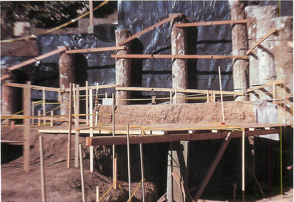
The piers exposed after drilling and pouring, and ready for forming the foundation and retaining wall between the piers
